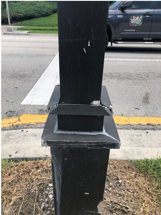
Figure 3.5-A– Typical Damage to Post Collars
